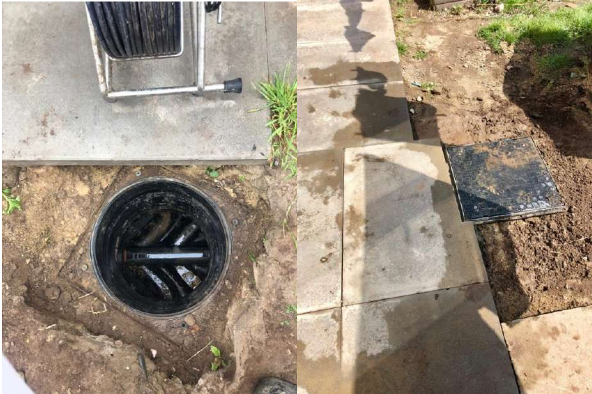
Manhole below ground level upon arrival.
